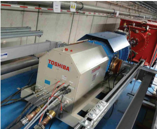
Figure 7: The first series MBK installed in the injector area of the European XFEL.
