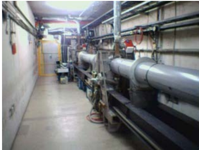
Figure 2.7: Inside Linac II tunnel.
